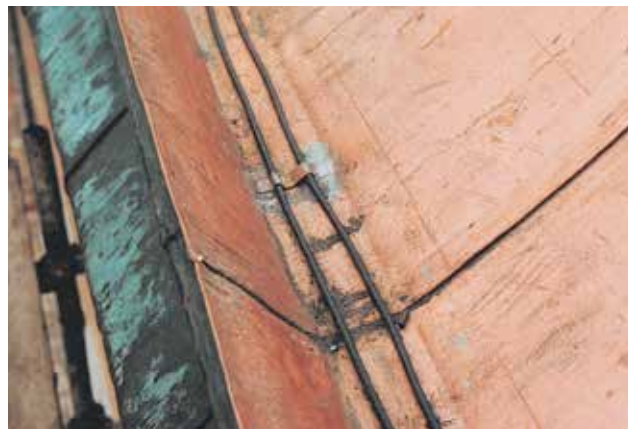
The formation of ice on the eaves can be prevented to some extent by using a heating cable, but it is important to design the roof initially in such a way as to prevent the formation of ice.
