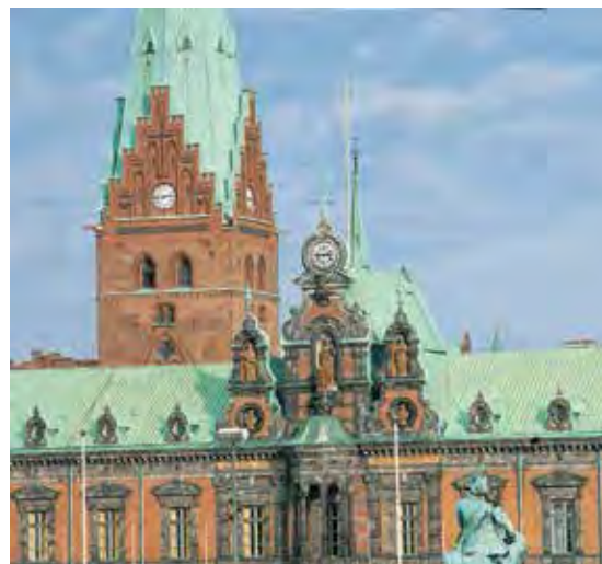
Copper roofs have an unbeatable lifetime. Nobody knows how old a copper roof can become. Malmö Town Hall, Sweden.
