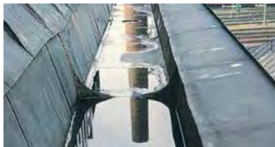
Blocked gulleys can result in major stresses on the roofing materials.
