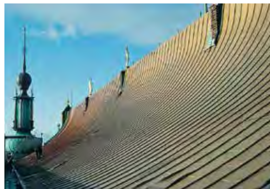
Correctly manufactured details and good maintenance are important criteria necessary to ensure that a roof does its job.
