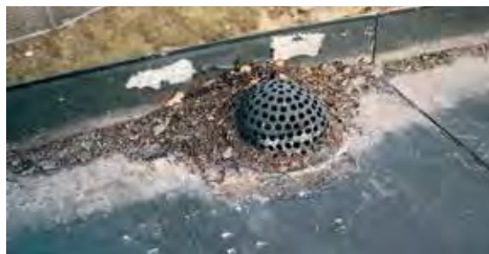
A gutter in which rubbish, leaves, etc. have gathered by a gully.
