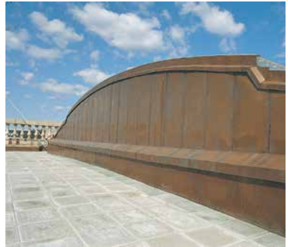
When terminating sheeting against high walls, the need for degree of movement must also be taken into account.
