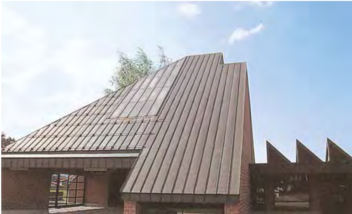
Attachment of a ridge rail with seam attachment which does not prevent the movement of the covering. There are a number of different kinds of seam attachments.
