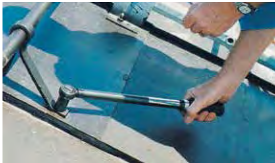
Roof safety device mountings in wooden bases must always be tightened. Lock joints, on the other hand, must not be tightened.
