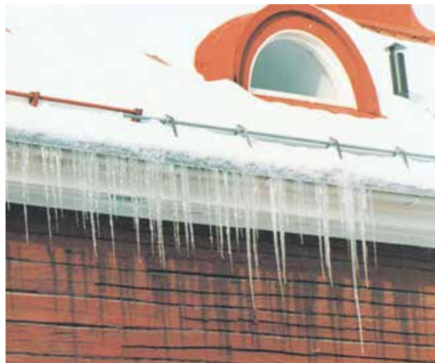
Icicles on the eaves indicate that heat is leaking out.
