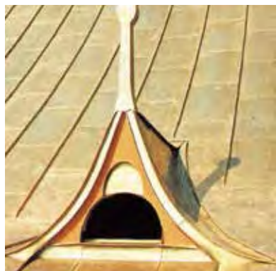
The flashing on details which are exposed to the wind must be checked, especially their fittings.
