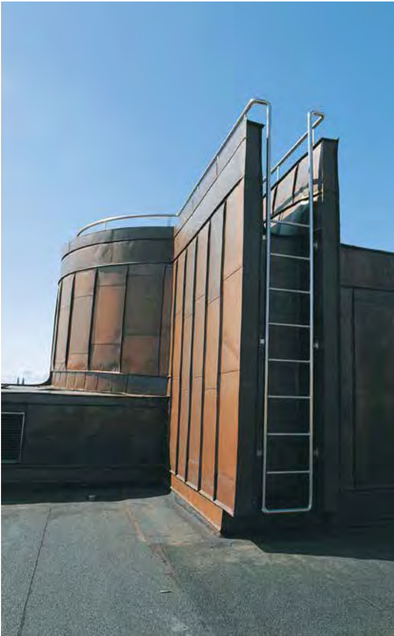
The best way to prevent damage as a consequence of accessing and working on the roof is to construct fixed walk ways.
