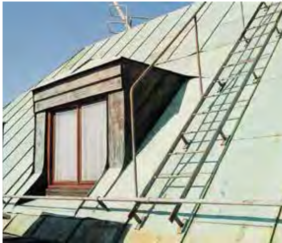
Checking the roof safety devices is a vital part of the maintenance inspection.
