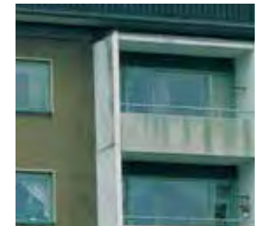
Water which contains copper can discolour pale surfaces and cause corrosion.
