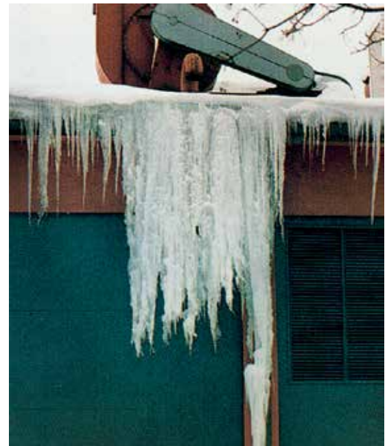
Errors in design or planning. The icicles indicate that there is insufficient insulation and /or defective ventilation.
